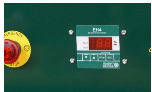
Panel-mounted EH4 in RL-71R.
